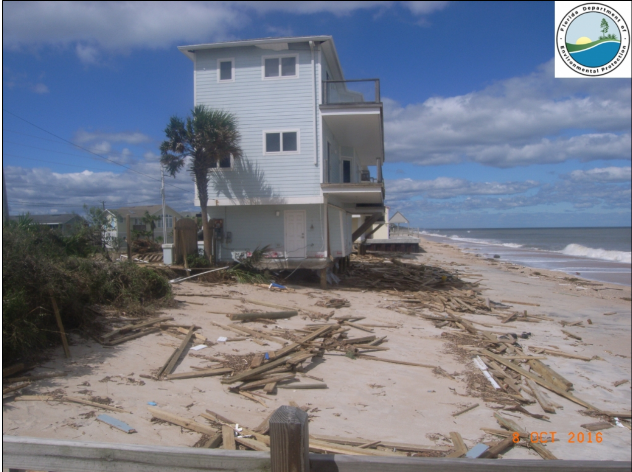
Figure 4-4. Hurricane Matthew damage in the vicinity of R114 on Oct. 8, 2016. Note erosion of sand below house. Image courtesy of Florida Department of Environmental Protection.
