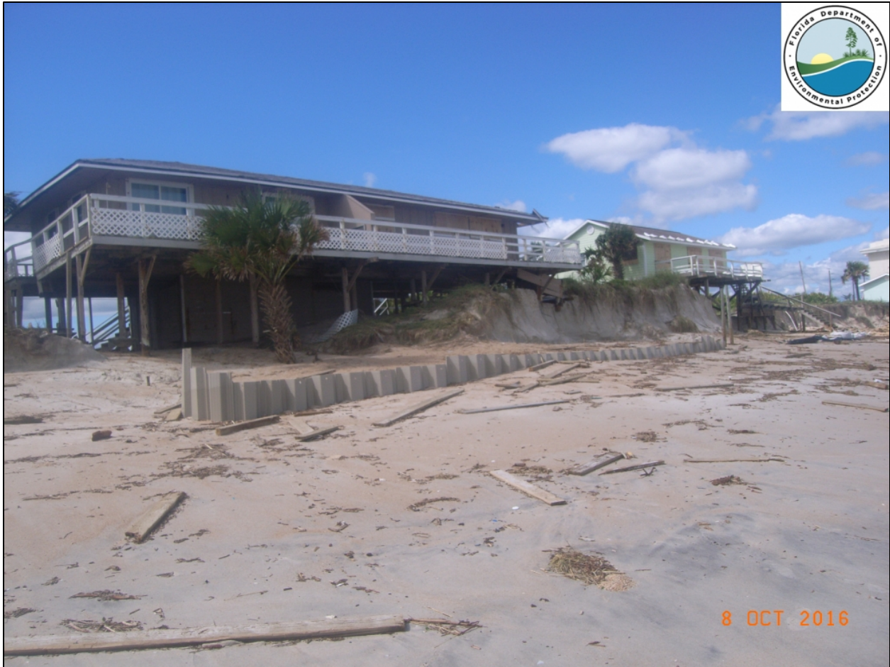
Figure 4-5. Hurricane Matthew damage in the vicinity of R116 on Oct. 8, 2016. Note top of vinyl sheet pile seawall emerging from sand in foreground and dune scarping and erosion below pile-supported homes. Image courtesy of Florida Department of Environmental Protection.
