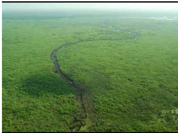
A view of the path cut through overgrown vegetation on Fisheating Creek by mechanical earth-moving machinery. Because the dredged material was sidecast into the waterway, it was determined to be a violation of Section 404 of the Clean Water Act, which prohibits dredge and fill activities in navigable waterways. (PHOTO FROM FLORIDA DEPARTMENT OF ENVIRONMENTAL PROTECTION WEBSITE)
