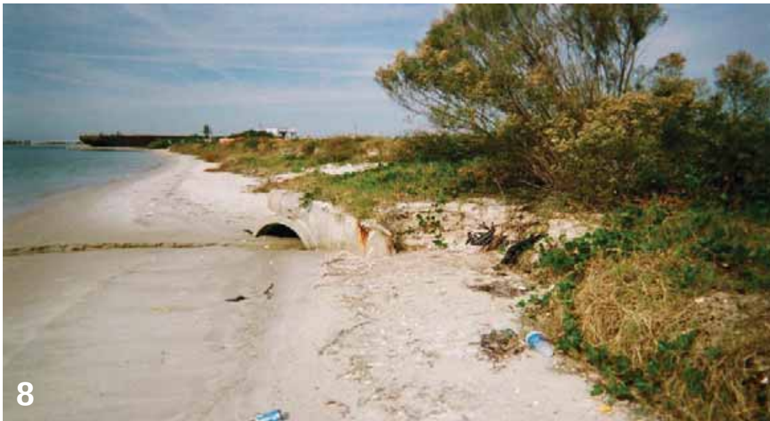
36-inch Stormwater Outlet (East of WTB)
