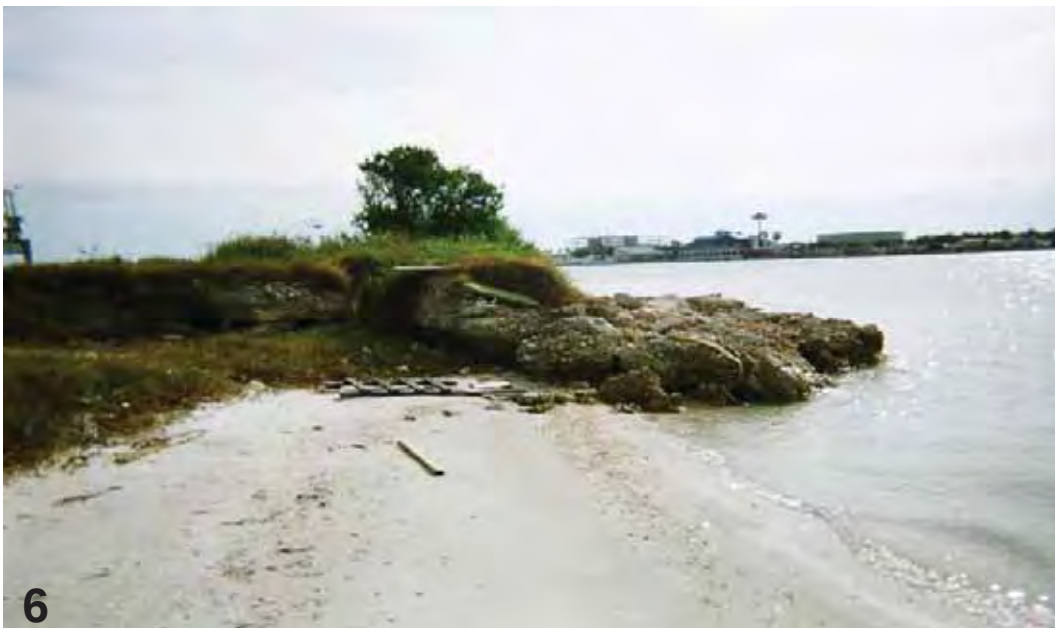
Rip-Rap East of WTB
