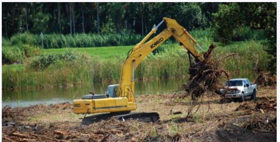
Land must be cleared of debris before filling the rock mining quarry, which will improve dike stability.
